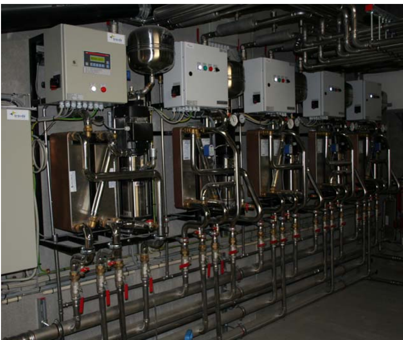
The mounted cooling units in the transmitting station in Videbæk
